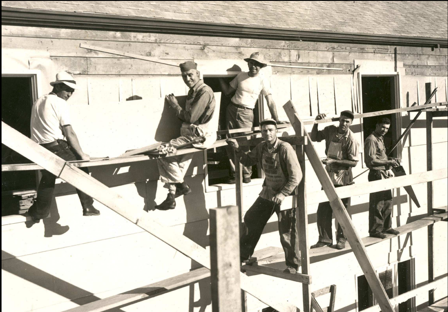
Building Crew - Unknown, Ernest Johnson, Pastor Gerlach, Art Wothe, Charlie McCullough, Mike Kukla.
